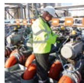
Page 113 Continuously challenging our systems and our processes Photo: Vopak Terminal Teesside (UK)
